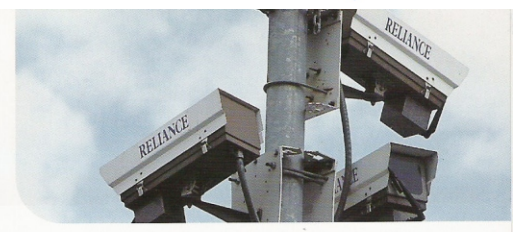
Typical application for type FPAS conduit and fittings includes security cameras.
